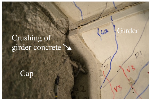
Figure 4.31: Crushing of girder concrete
