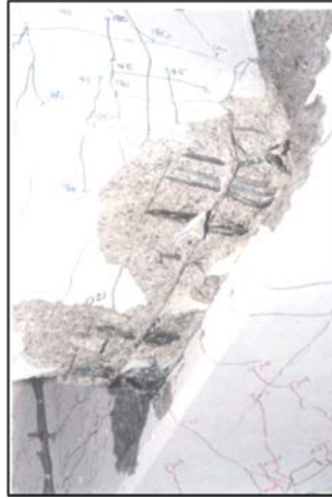
Figure 2.11: Spalling of bathtub girder at cap interface (Holombo, 1999)
